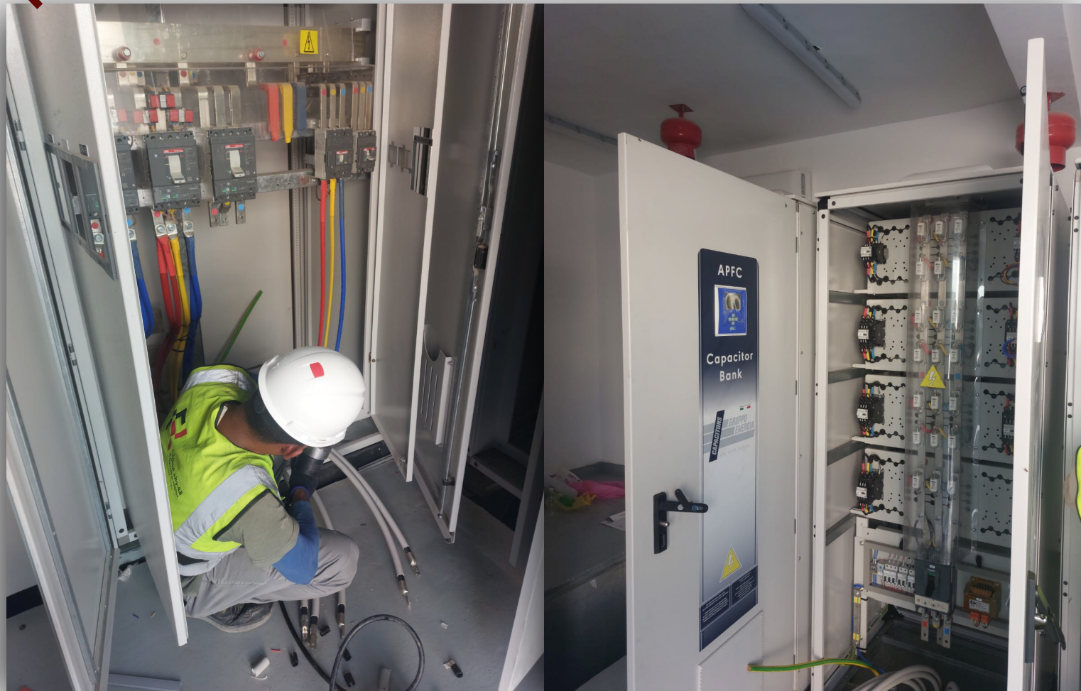
Power Factor Correction System Installation – Al Habib Factory
